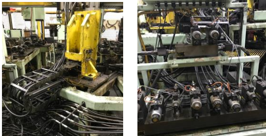
Previous system, a mess of hydraulic components
